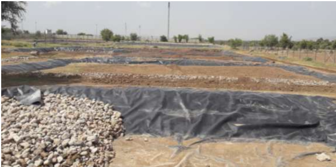
Picture 8: Overview of PW Treatment Plant
