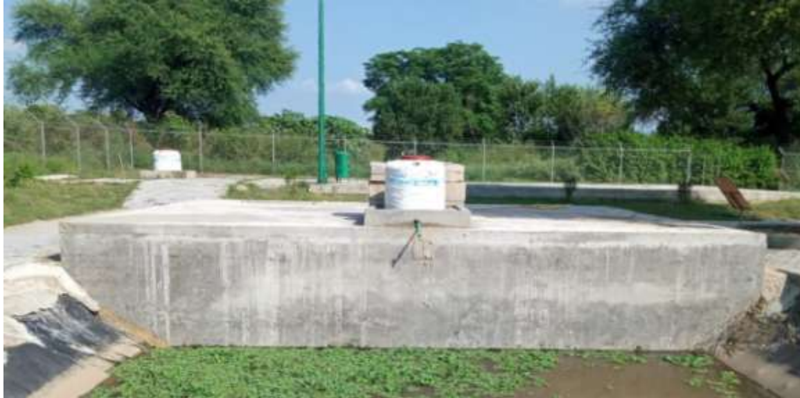
Picture 1: Ext. ABR and Bio gas incinerator
