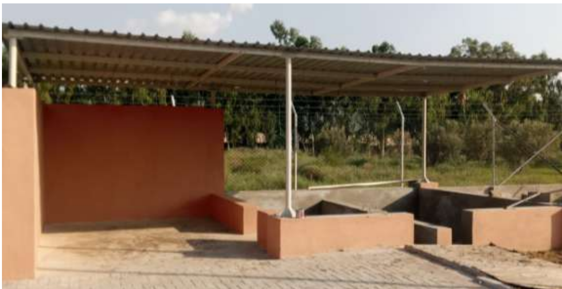
Picture 4: Slurry Outlet bed + Compost Storage Shed
