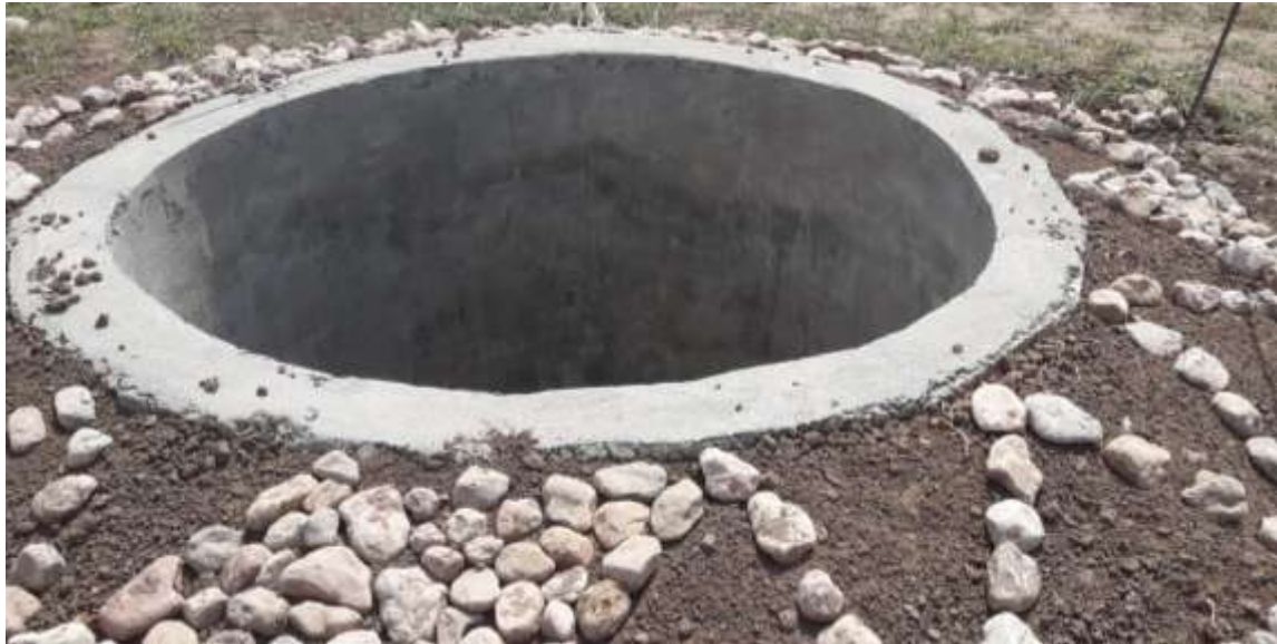
Picture 7: Water Collection Tank
