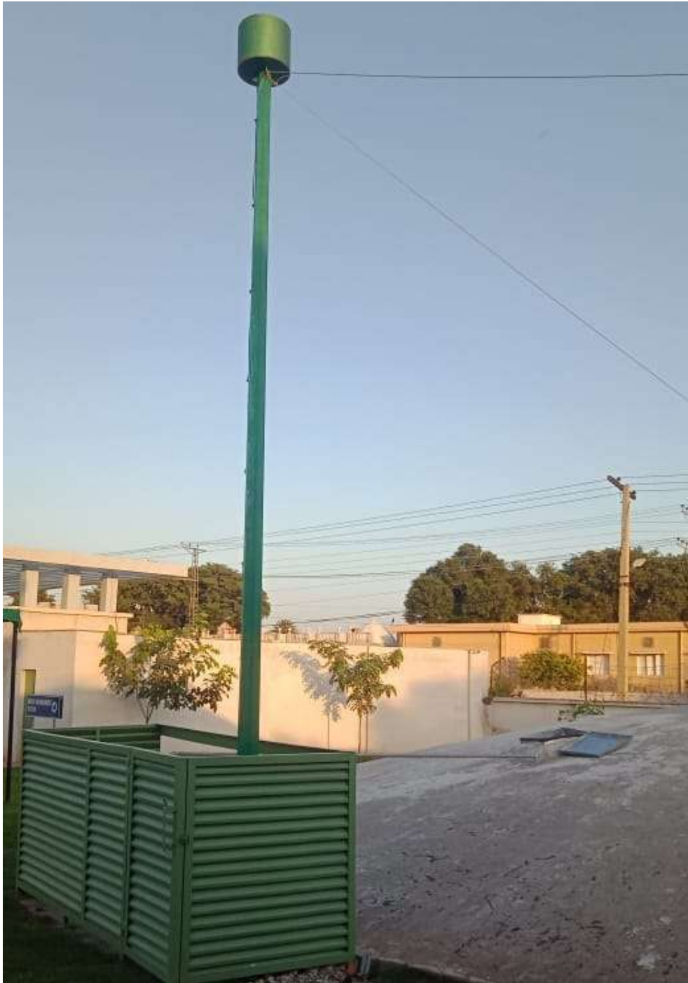
Picture 3: Bio-Gas Incinerator
