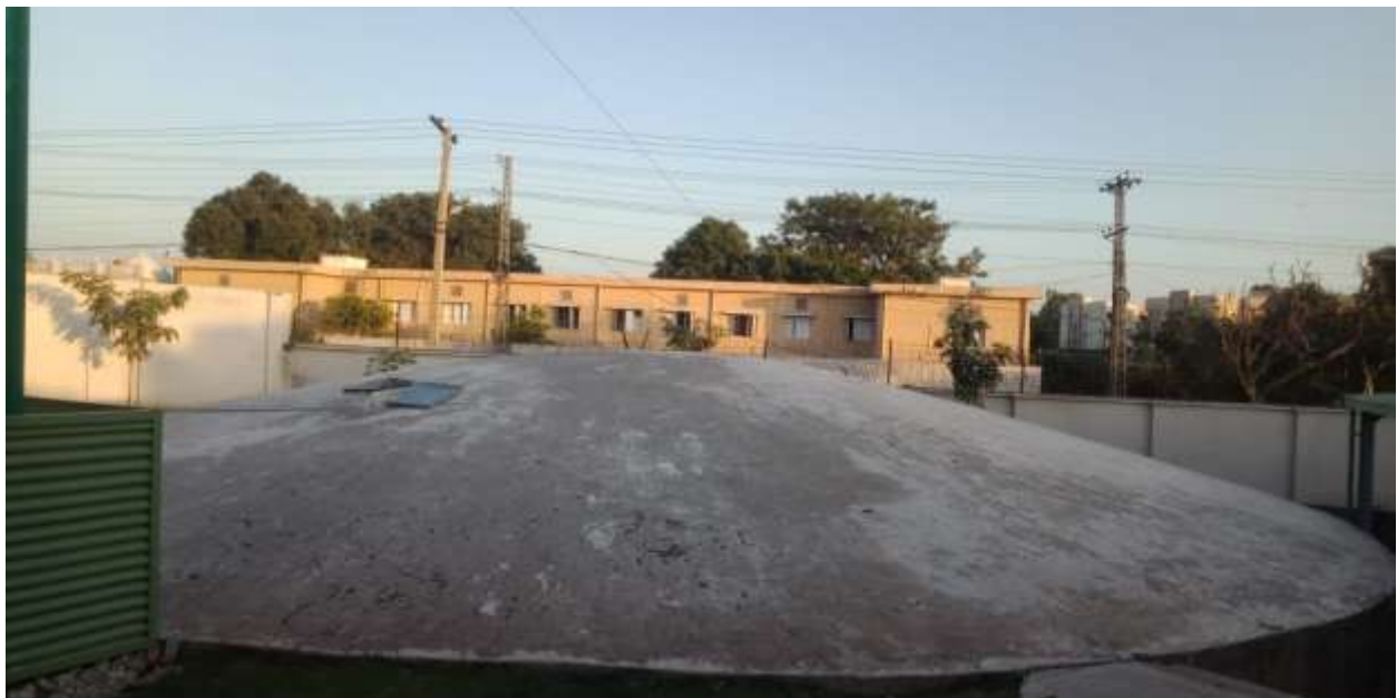
Picture 2: Bio-Digester Tank
